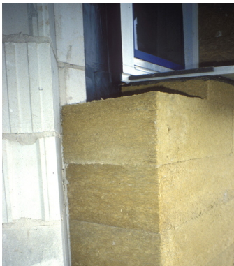
Figure 31: Photo of the 40 cm insulation material (mineral wool) at the “Ultrahaus” in Rottweil, Germany.
