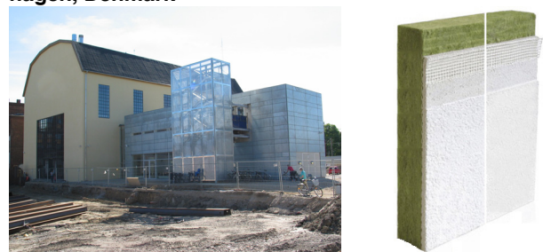
Figure 71: Photo of the cultural centre Proevhallen in Copenhagen (left), and the system chosen for the application at the external wall (right, www.rockwool.dk ).
